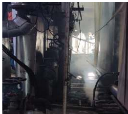
Figure 8: Steam Leak from Piping
